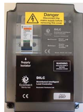
DILC in wall mounting enclosure as installed on Island of Foula, Scotland (also available as DIN-rail type)
