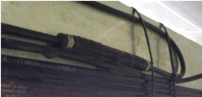
Fig. 9: Fastening of the connector tight to the mounting structure can cause moisture build up between connector and rail, damaging the connection
