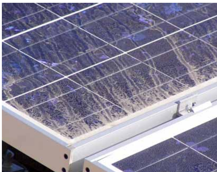
Fig. 2 Dust fall on solar panels.
