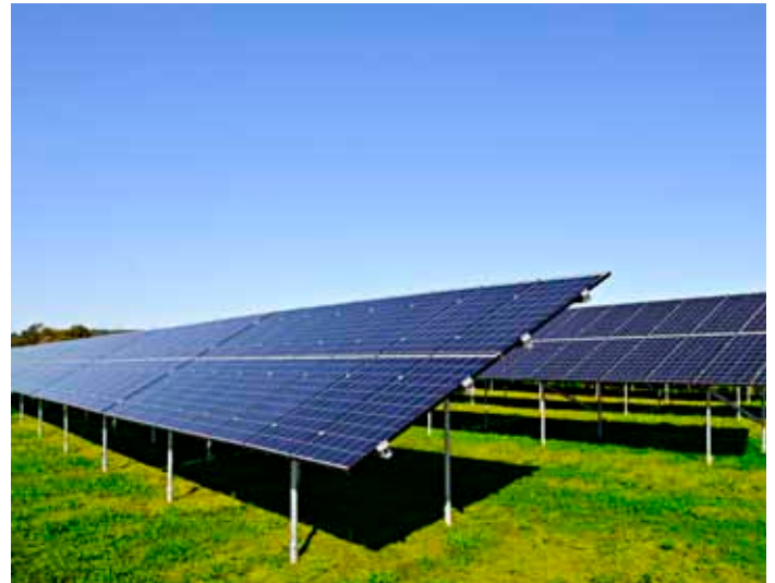
Fig. 3: A clean and functioning solar installation
